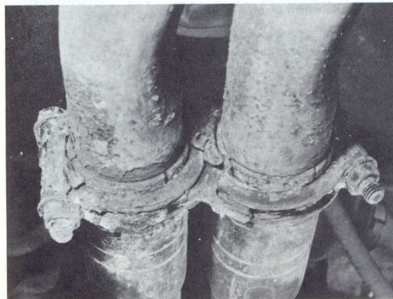
27.6B Exhaust system intermediate joints
